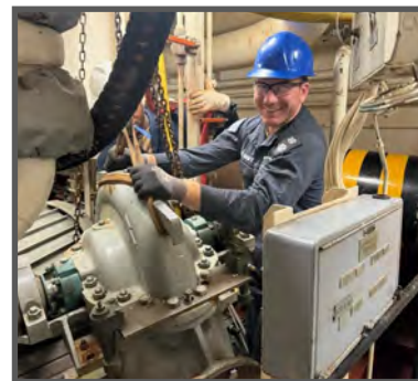
USS Carney's (DDG 64), BM2 Joshua Pennington assists in the alignment of No. 5 Sea Water Service Pump. (Photo by IT1 (IW) Andrew Cole.)
