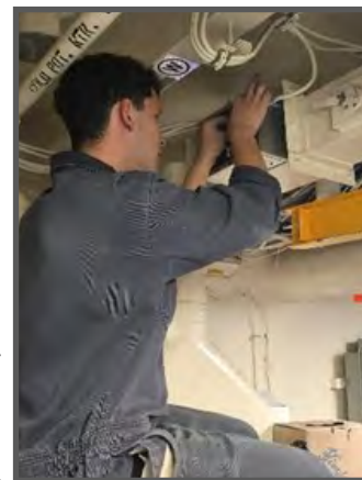
EM2 Daniel Cerrato conducting a solenoid repair on a vent dampener in the rewind shop aboard USS Anchorage (LPD 23). (Photo by Rizalito Antonio.)
