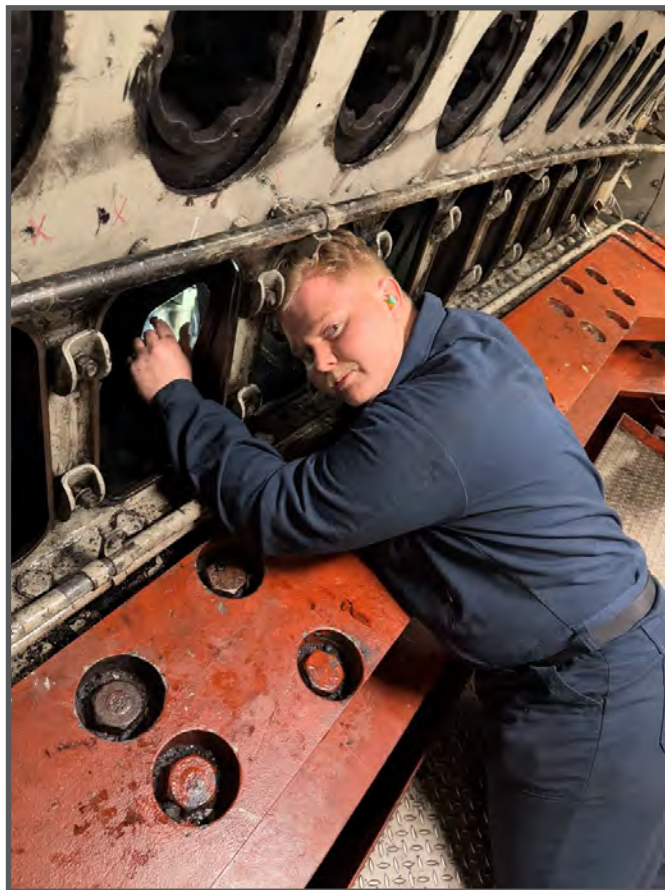
EN2 Bleize Parker assisting in a Diesel Engine Inspection on Number 1 Ship's Service Diesel Generator aboard USS Harpers Ferry (LSD 49). (Photo by EM1 (SW) Seth Waers.)
